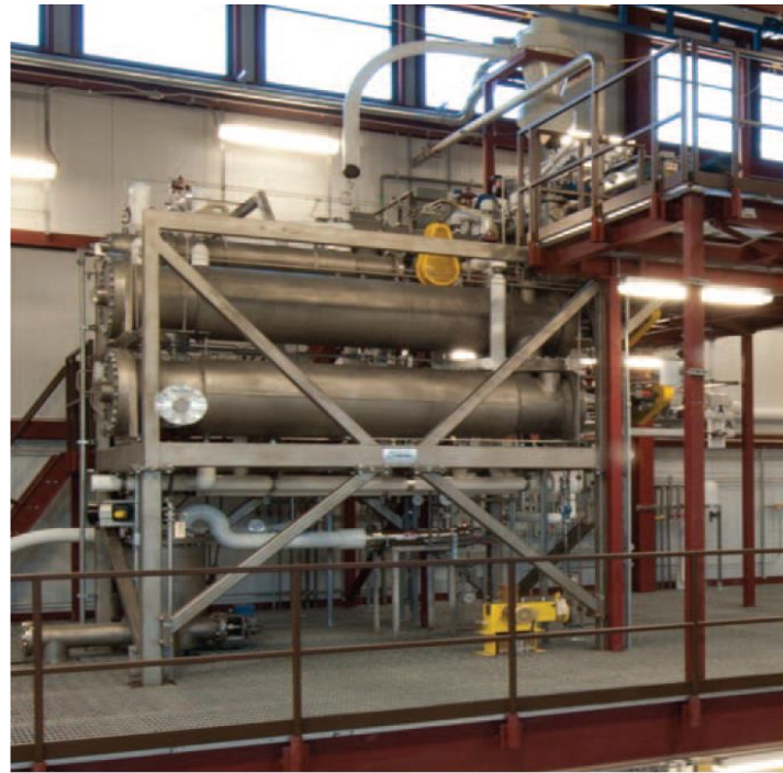
Photo by Dennis Schroeder, NREL/PIX 17684
