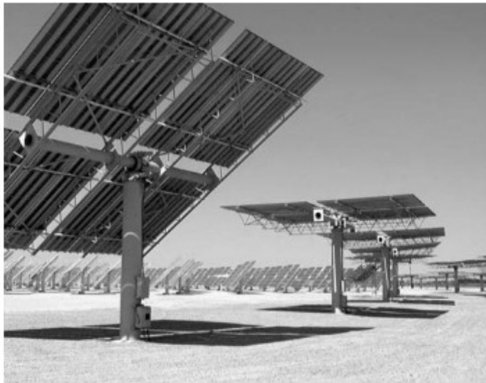
FIGURE 3.22 Detail of a heliostat.
