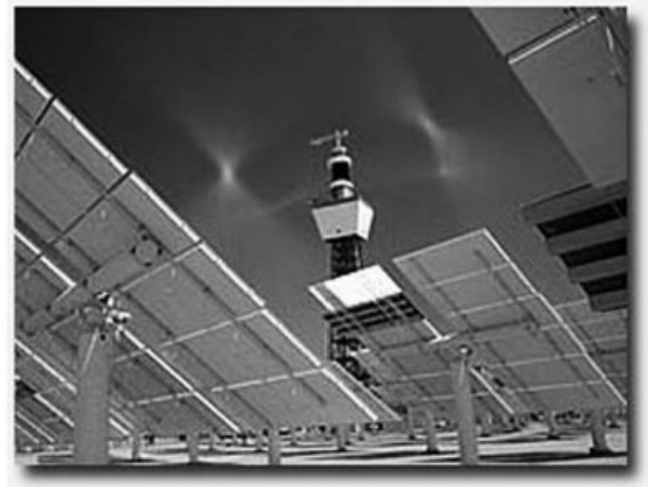
FIGURE 10.7 Heliostat detail of the Solar Two plant (source: www.energylan.sandia.gov/sunlab/overview.htm ).
