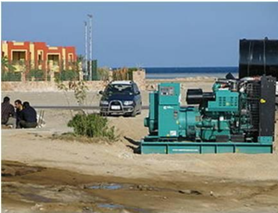
diesel generator in Egypt
