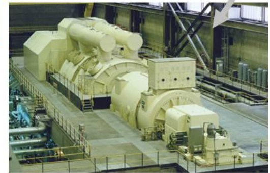
steam turbine generator
