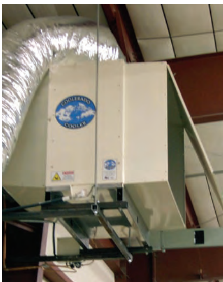
Figure 12. Coolerado Cooler test unit at NREL's Thermal Test Facility. Source: NREL
