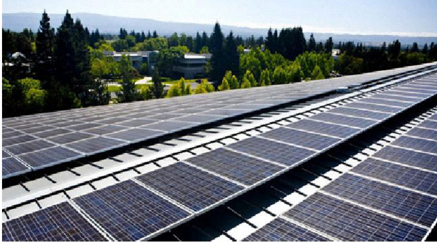
Figure A.3 A view of solar collectors [2].
